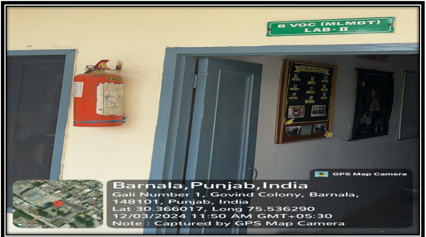
Fire Extinguishers in Campus to ensure safety and security
