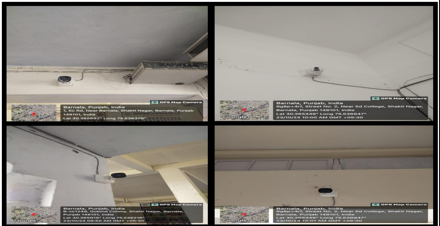
CCTV camera's at various point in the campus
